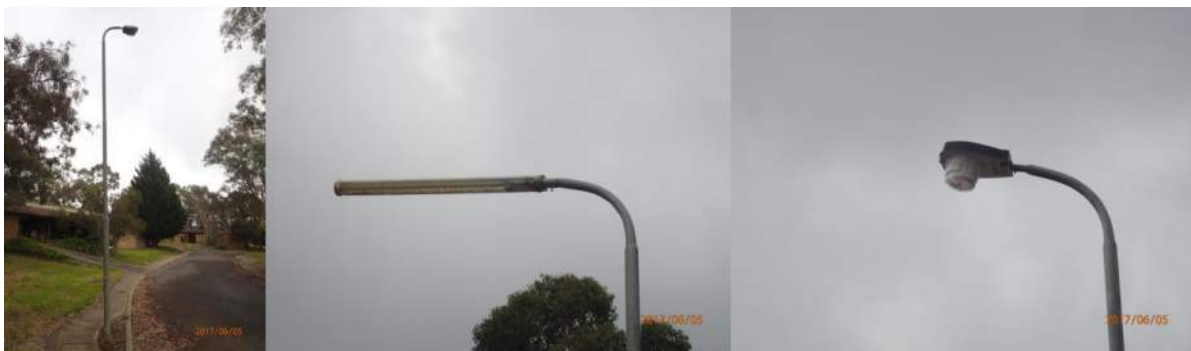
Figure 2.8 – Street Lighting Fixed to Stand-alone Poles
