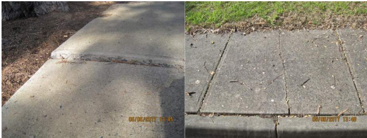
Figure 2.5 - Typical Footpath Defects
