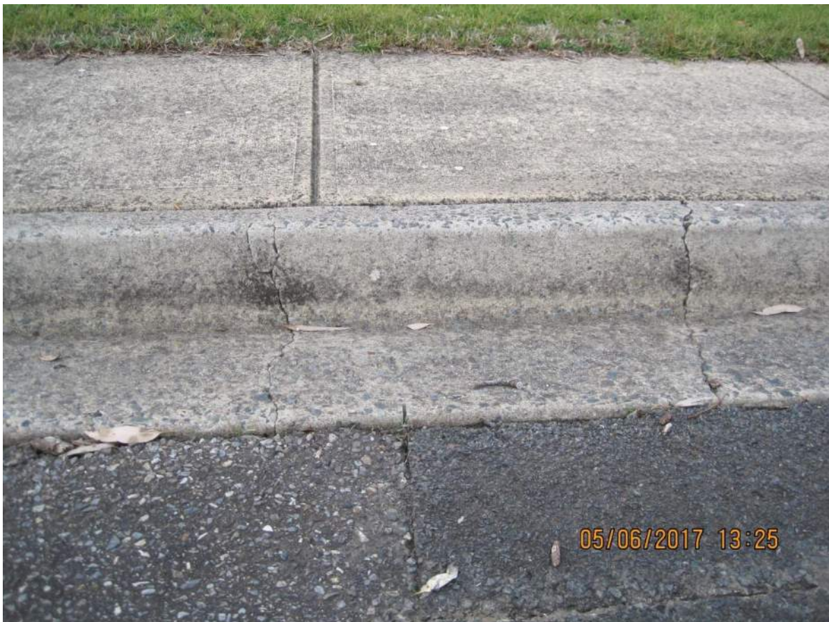
Figure 2.2 – Typical 'Type 1' Kerb Condition & Geometry (Appendix B, Photo 12)
