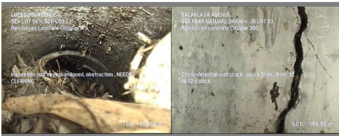
Figure 2.10 - Various Blockages and Cracks Found Through Investigation
