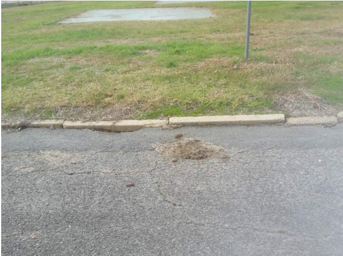
Figure 2.4 – ‘Type 3’ Kerb Condition & Geometry (Appendix B, Photo 365)
