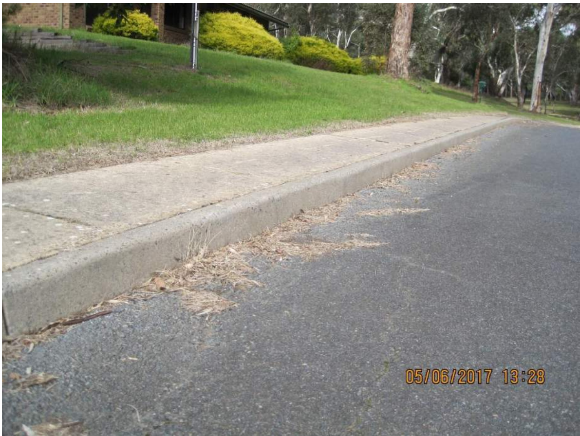
Figure 2.3 – 'Type 2' Kerb Condition & Geometry (Appendix B, Photo 20)
