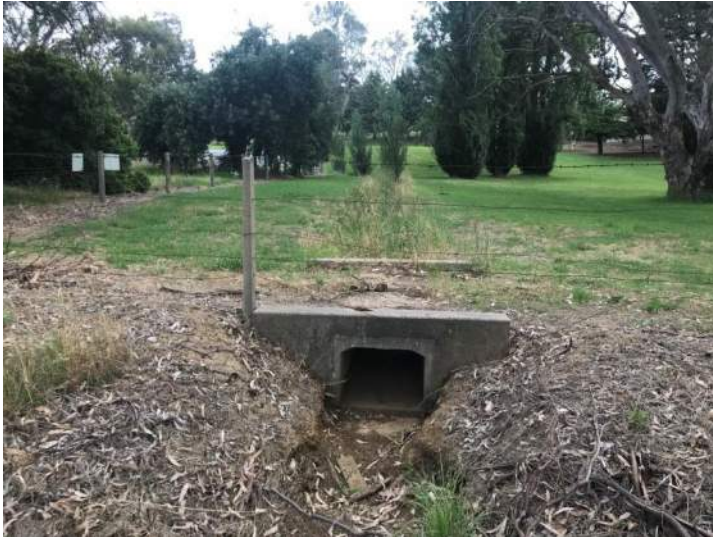
Figure 5: Headwall Outlet from Creek Catchment to Roadside Swale (looking south from road)
