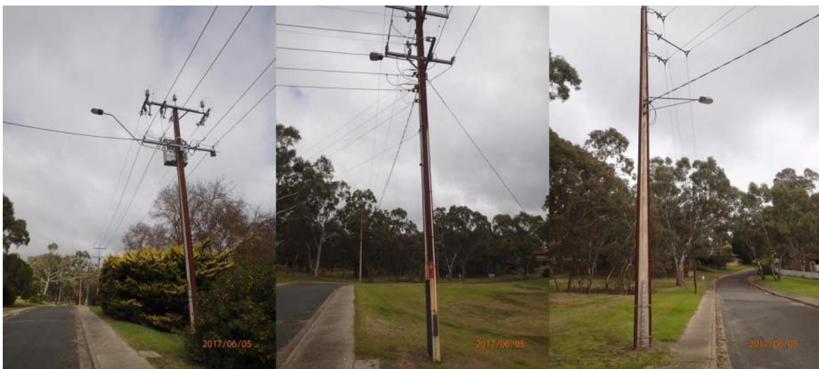
Figure 2.7 – Street Lighting Fixed to Stobie Poles
