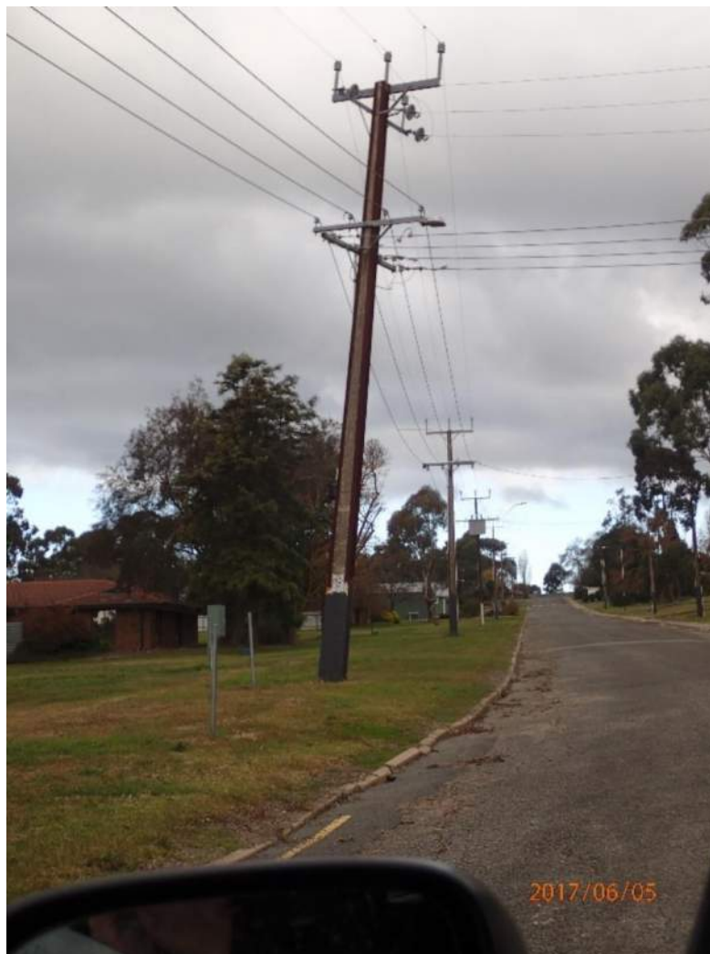
Figure 2.9 - Leaning/Slanting Stobie Pole (Appendix D, Photo 41)
