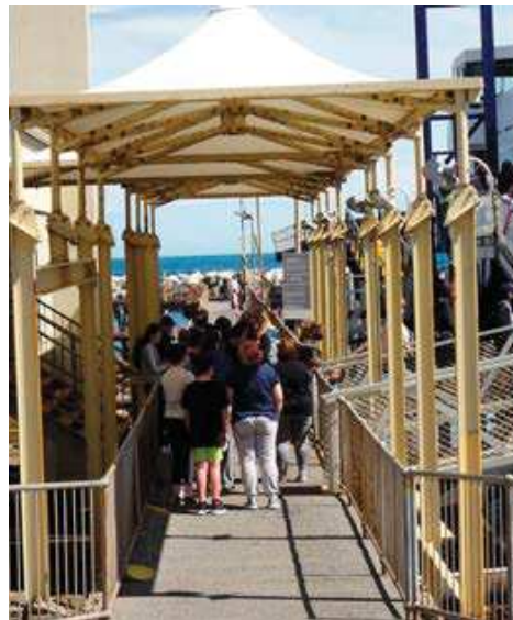
The current jetty with a shade structure and ferry access are all showing signs of deterioration that detract from the visual amenity
