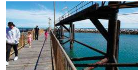
The jetty is coming to the end of its useful life
