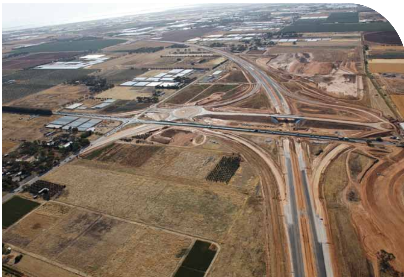
Above: A view of intensive construction works at the Heaslip Road Bridge and Womma Road interchange where it connects with the Northern Expressway.
