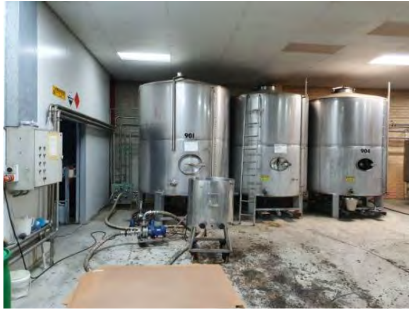
Photograph 7- View of the vinegar plant storage tanks, pump and corroded concrete flooring.
