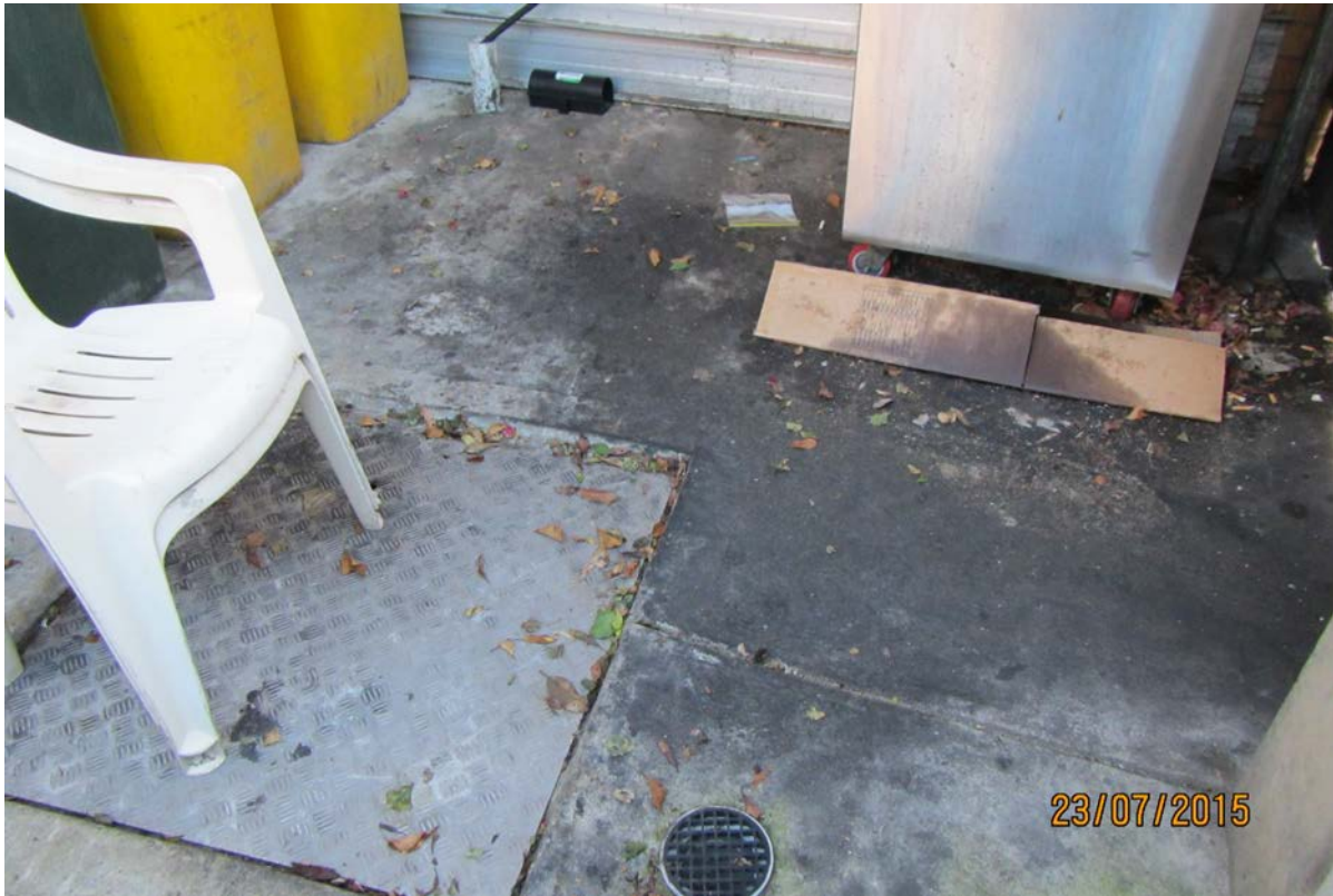
Photograph 3: Grease Arrestor adjacent to kitchen facilities.
