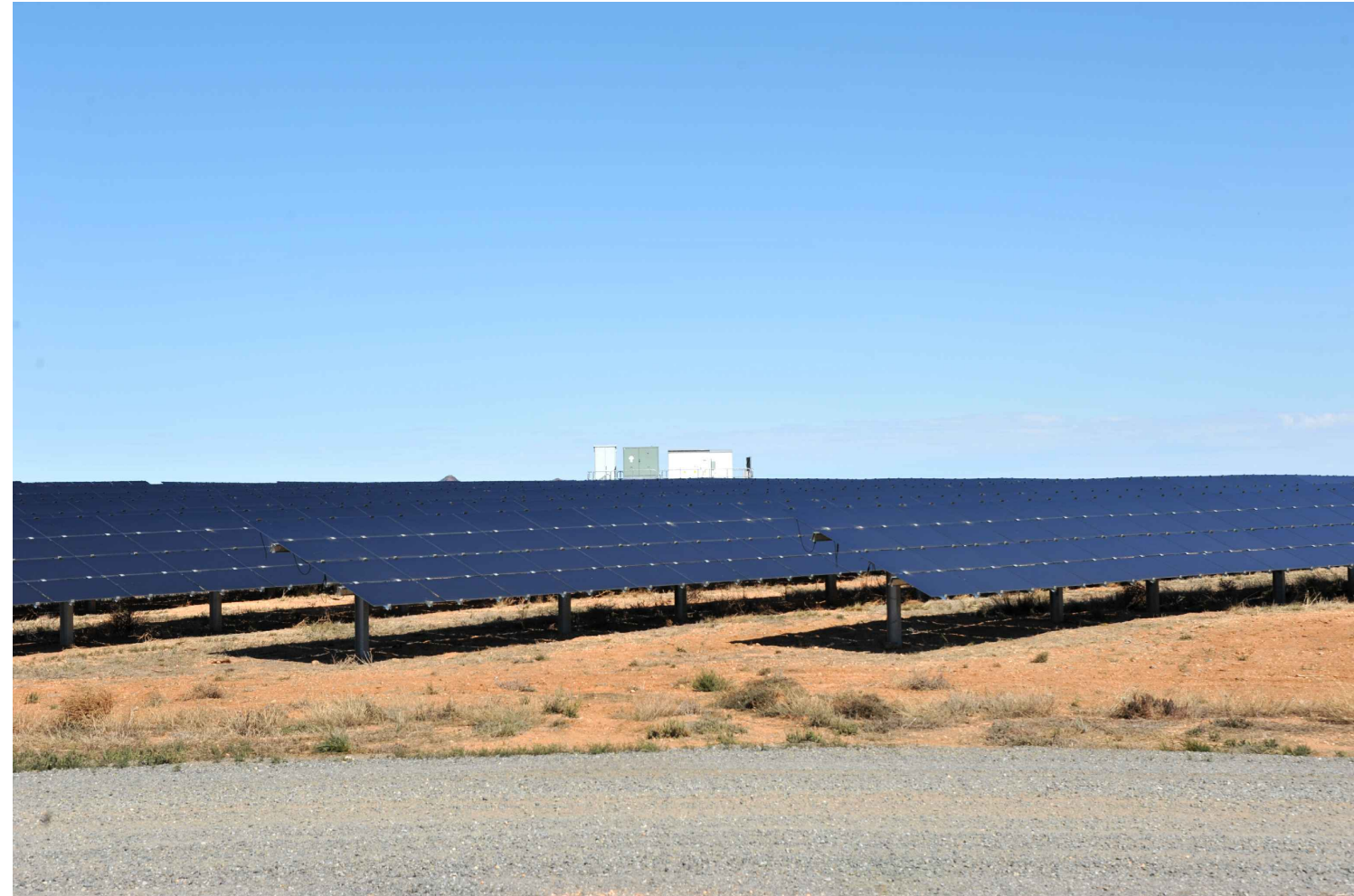
Plate 4 - Typical detail view toward photo voltaic panels and inverter units
