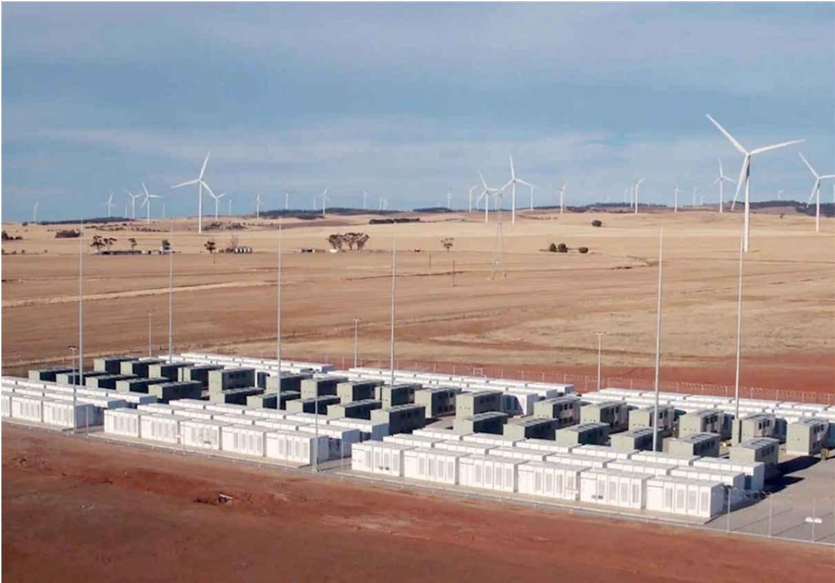
Plate 1 – Typical battery storage facility, Hornsdale SA (Image: Neoen Australia Pty Ltd 2017)
