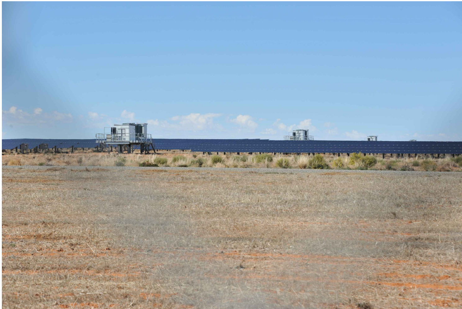
Plate 1 - Typical view toward photo voltaic panels and inverter units
