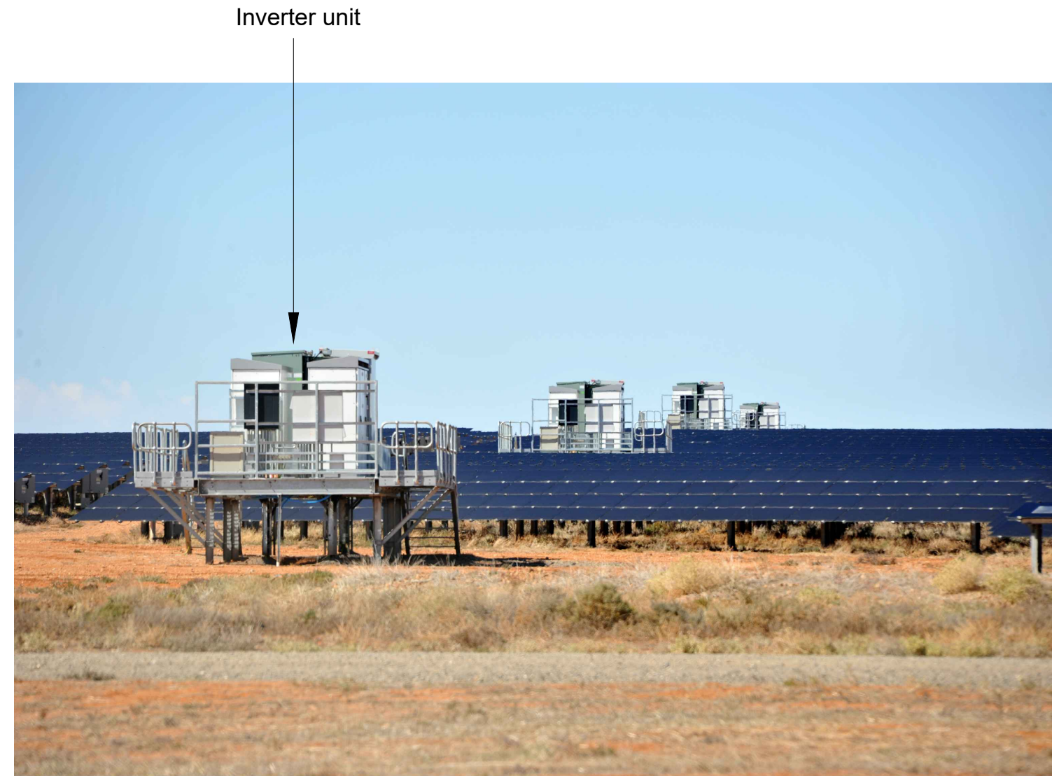
Plate 2 - Typical detail view toward photo voltaic panels and inverter units
