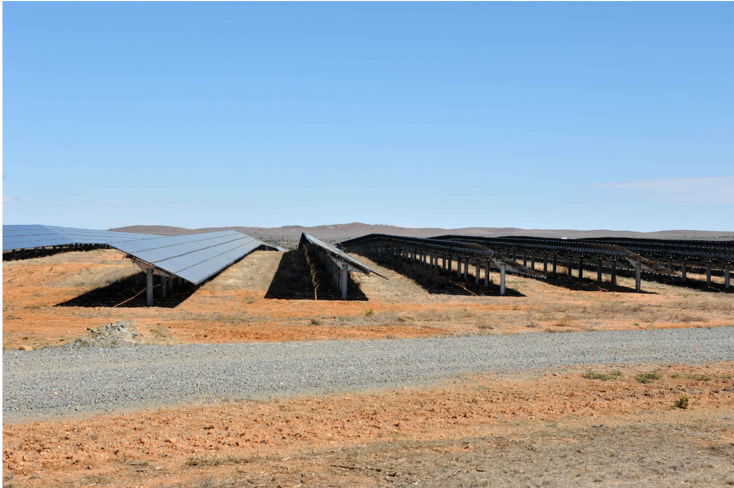
Plate 3 - Typical view toward photo voltaic panels (single axis face and underside)
