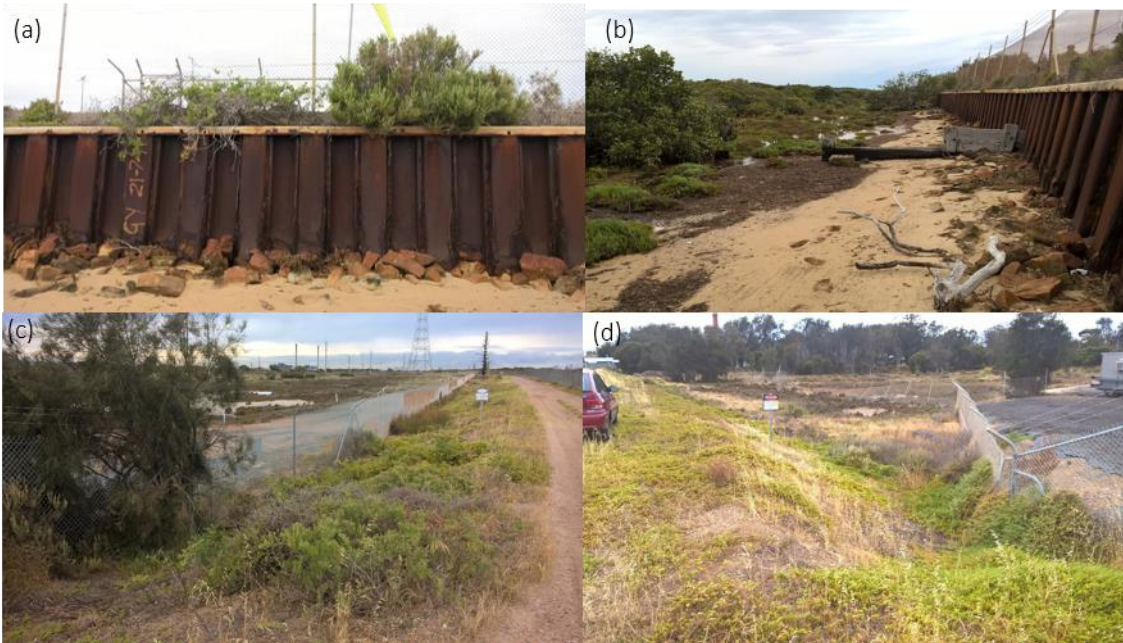
Figure 9: HDD is expected to have no impact on (a) the seawall (b) fringing mangroves (c) access road and (d) existing gas owners using the easement.
