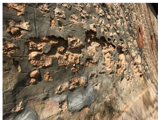
Example of the deterioration of stone as a result of hard cement pointing.
